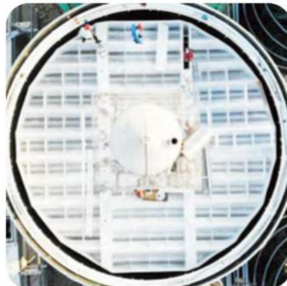
Three-Phase Separator (GLSS)
